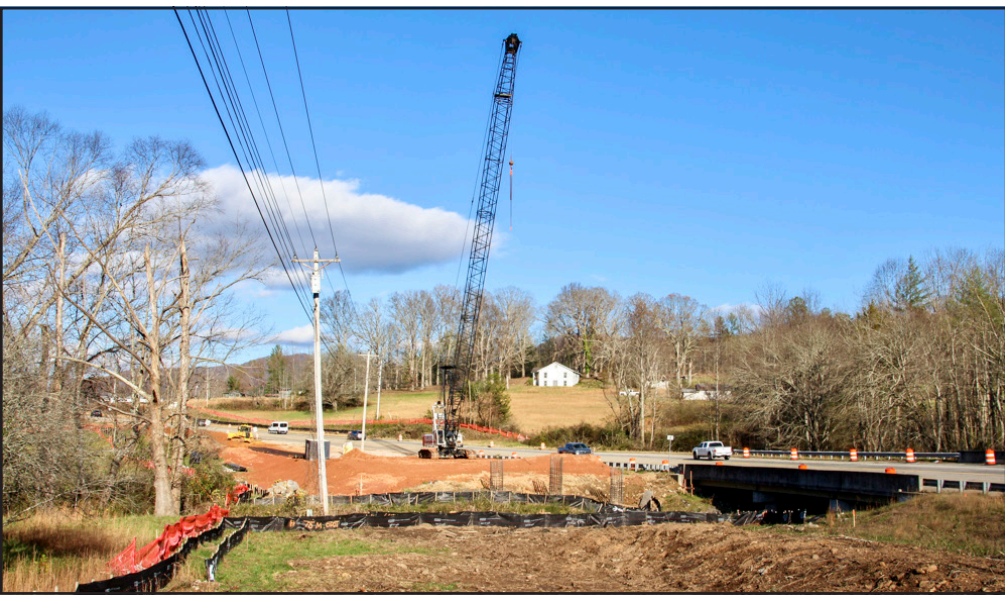
Construction of the new bridge over Brasstown Creek at the county line continues apace as part of the GA 515 project.
